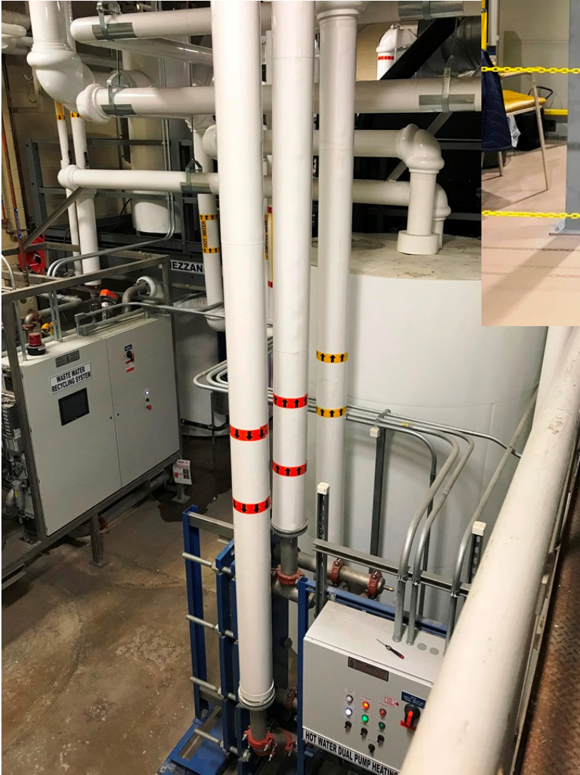
Heat Recovery System and Storage Tanks
